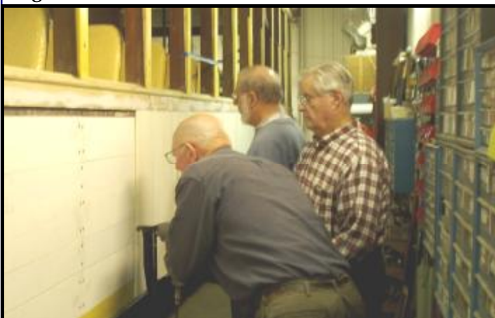
Men at work! Here we see (from left to right) Ken Albrecht, Phil Settergren and Dick Stoner installing the tongue and groove siding (sometimes called "wainscoting") on the "pole side" of No. 1300. (John Prestholdt photo)
