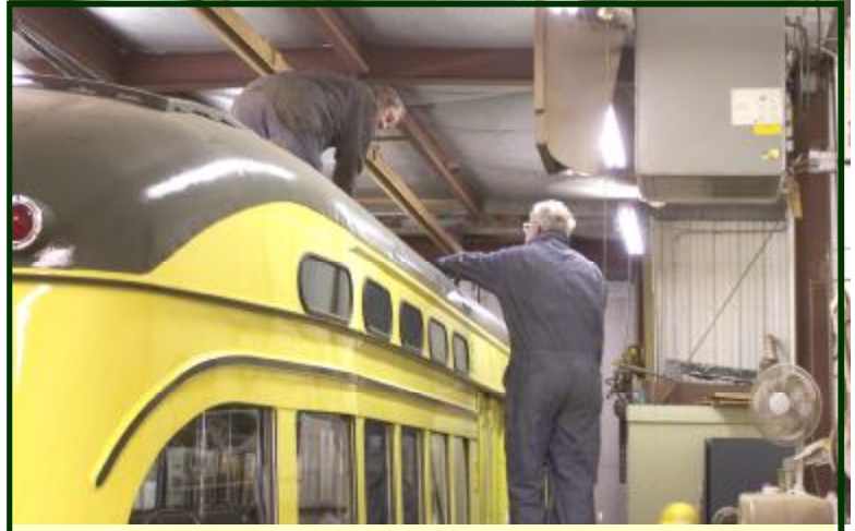
Where are those pesky leaks? Jim Willmore is on the roof of PCC No. 322 and he is ably assisted by Neil Howes on the ladder as they go about the task of finding and repairing a few leaks on No. 322’s roof. (Jim Vaitkunas photo)
