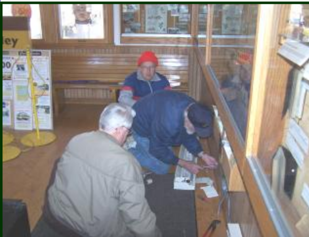
Men at work! Here we see (from top to bottom) Russ Isbrandt, Keith Lindberg and Dick Stoner installing the electric baseboard heater in the Linden Hills station. (Jim Vaitkunas photo)
