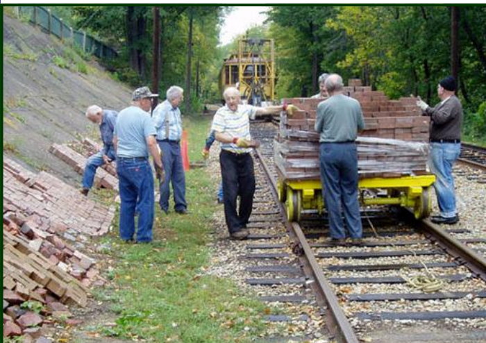
There's always something to do at the Isaacs car barn. Here we see the bulk of the "Tuesday crew" stacking bricks on the west retaining wall in front of the Isaacs car barn. These bricks were formerly used for our platform at the Linden Hills station. From left to right are Walt Strobel , Roy Harvey , Neil Howes , Russ Isbrandt , someone behind Russ, Mark Digre , Phil Settegren (back towards us) and Jim Otto . Others that helped with the work include Scott Heiderich , Bill Arends and John Prestholdt . (John Prestholdt photo)
